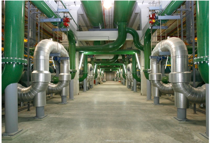
District Cooling Plant supplies chilled water to the Burj Khalifa and Dubai Mall.
