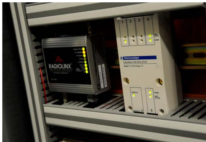
ProSoft Technology RadioLinx industrial Ethernet radio & Schneider Electric ConneXium 499 NES 25100
