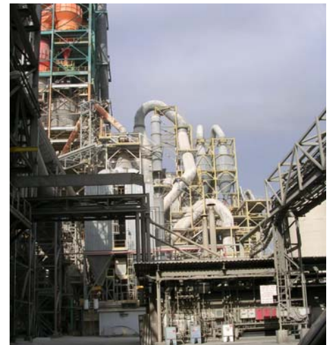
Nesher Cement Plant, Israel
